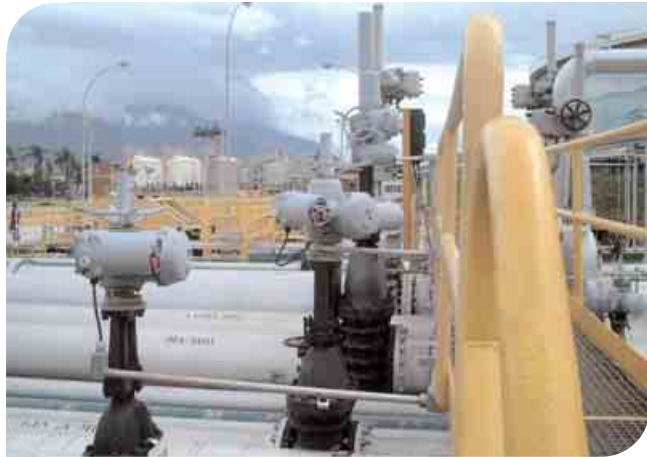
ST INTELLI+ Oil terminal (Brazil)
